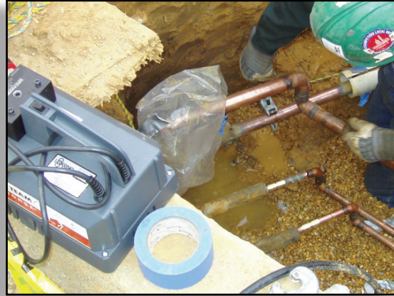
This outside installation used LOKRING couplings to connect existing medical gas lines to new lines for hospital expansion. The completed installation included 3/4" size for nitrogen and nitrous oxide. The oxygen line was 1 1/2" size on Type L copper. The total installation time for the three fittings was 20 minutes.
